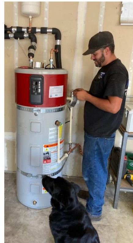
120-volt HPWH installed as part of NBI's California field study
